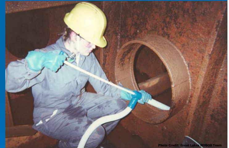
Pumping residual water with a hand-operated pump in a double bottom ballast tank.
