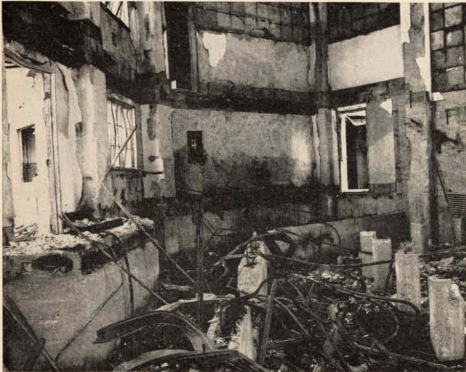
REINFORCED CONCRETE BUILDINGS STILL STAND —but note how the interiors, as in the operating room of the Nagasaki University Hospital (2,200 feet from ground zero), are burnt out. Fire has consumed the floor, the balcony, and all seats, and distorted the metal railings and pipe.
