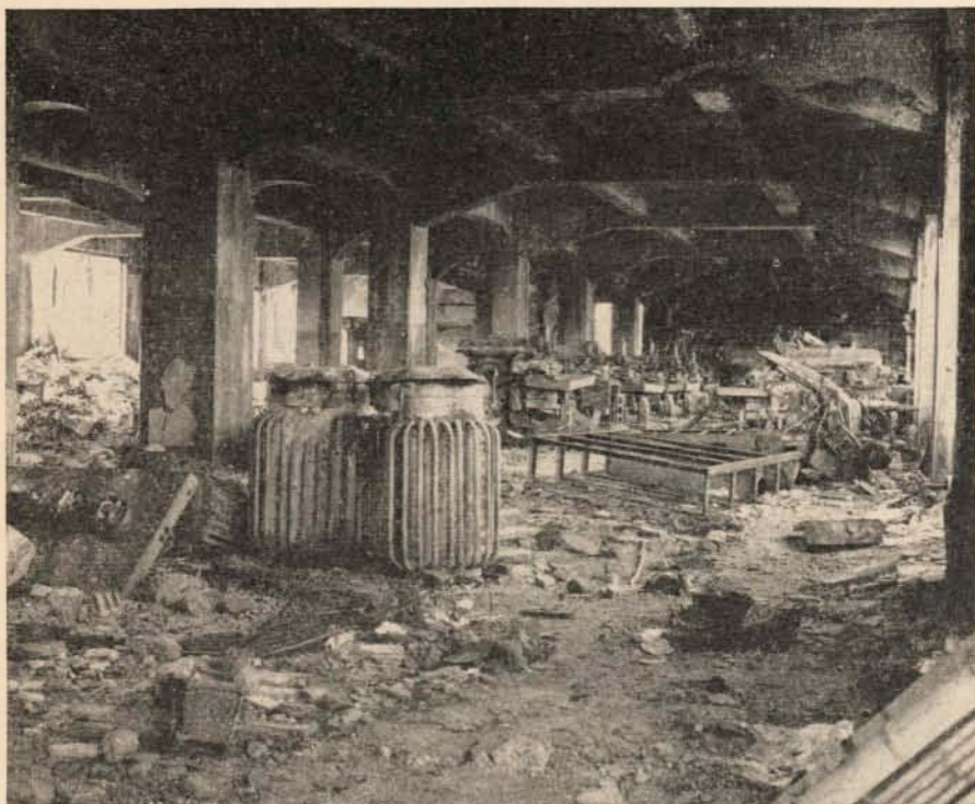
BLAST STRUCK DOWNWARD against the roof of the Chinzei School, 1,500 feet from ground zero at Nagasaki, which had been taken over in part for munitions work. The fourth story collapsed completely, but the heavy earthquake-resistant structure protected some machine tools on the first floor from serious damage. Electric transformers and a switchboard did not escape; a combination of blast, fire, and debris destroyed them.
