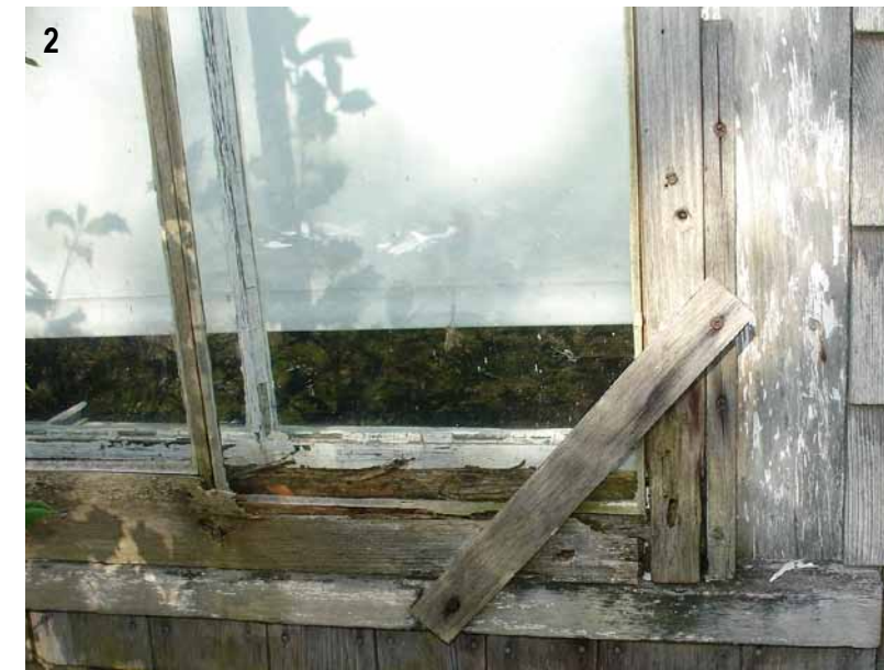
1. South porch roof needs to be reattached to main structure.
