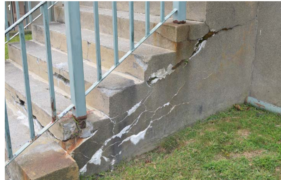
1. The front stairs exhibit significant cracking and loss of concrete. The railings show rust and paint loss.
