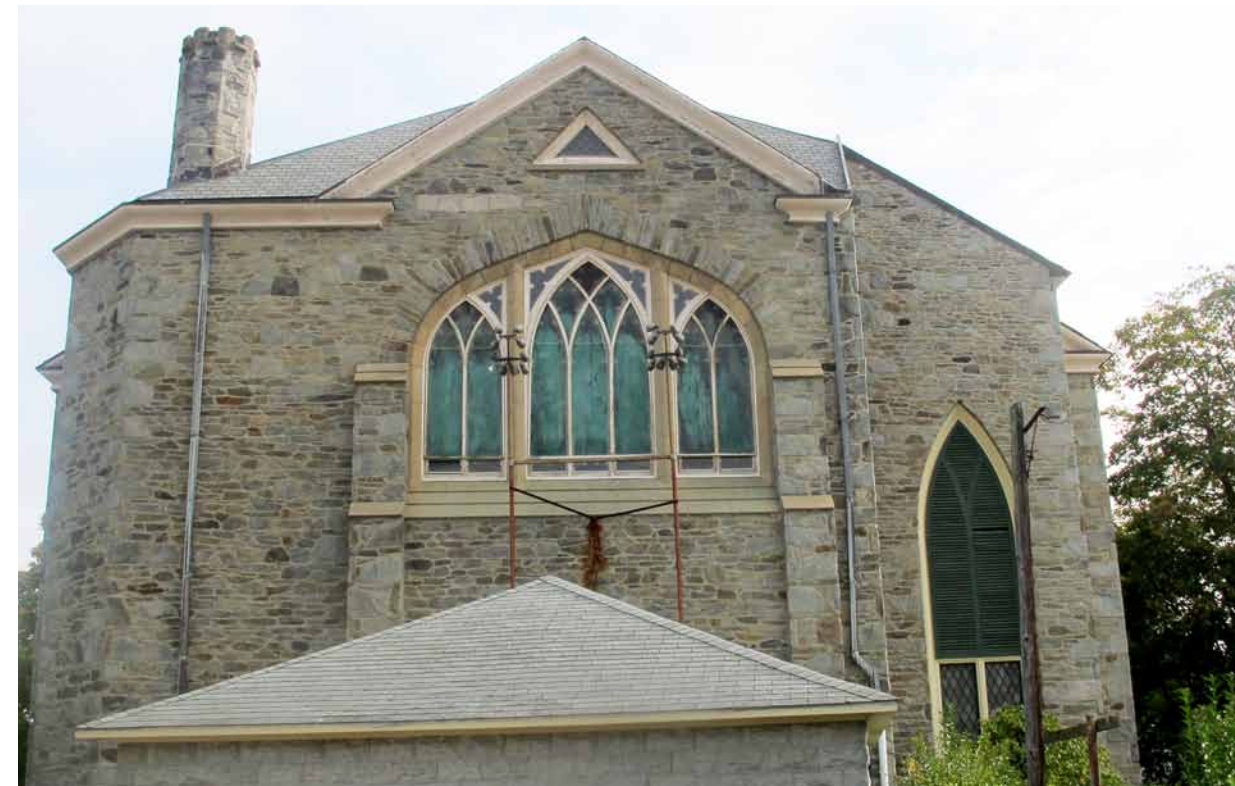
West elevation shows some stone wall rust staining, which needs to be cleaned.
