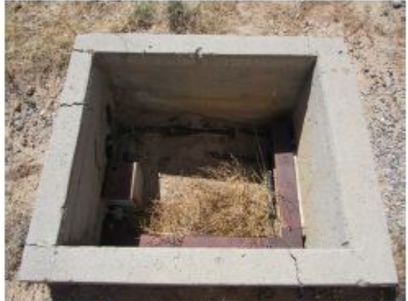
Overview of concrete pull box associated with Building 27110
