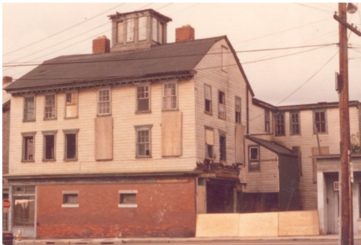
Figure 25: Photograph of the John Coddington House in a dilapidated state, circa 1970s. Courtesy of The Newport Restoration Foundation.
