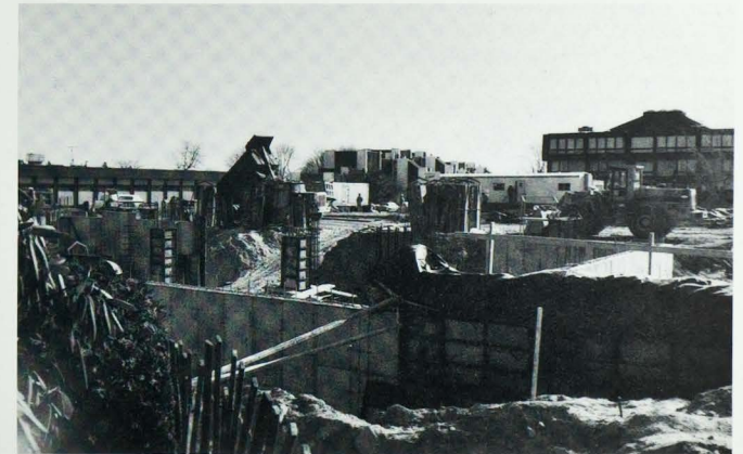
By mid-December 1989, the basement foundation of the new Library had been poured and the forms partially stripped.
