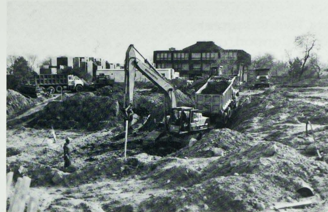
In early November 1989, excavation of the basement foundation for the new Library was underway.
